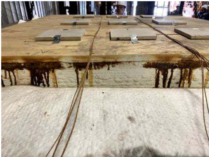
Photo No. 18 Assembly framing bubbling
