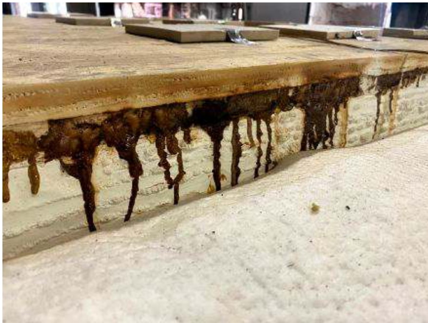
Photo No. 16 More moisture escaping
